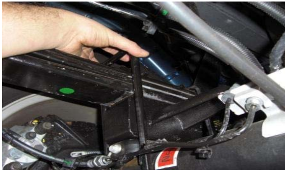
15. Replace u-bolts over leaf spring and axle.
